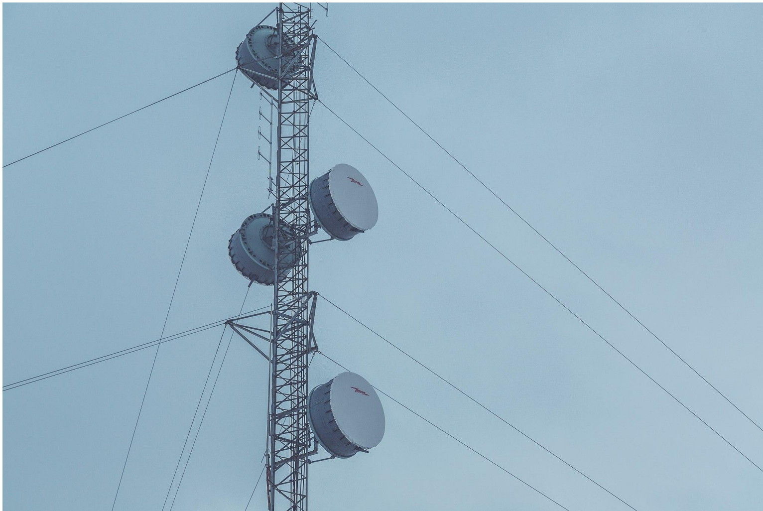
By Tony Webster BNSF Communications Tower CC BY-SA 2.0 Wikimedia Commons
